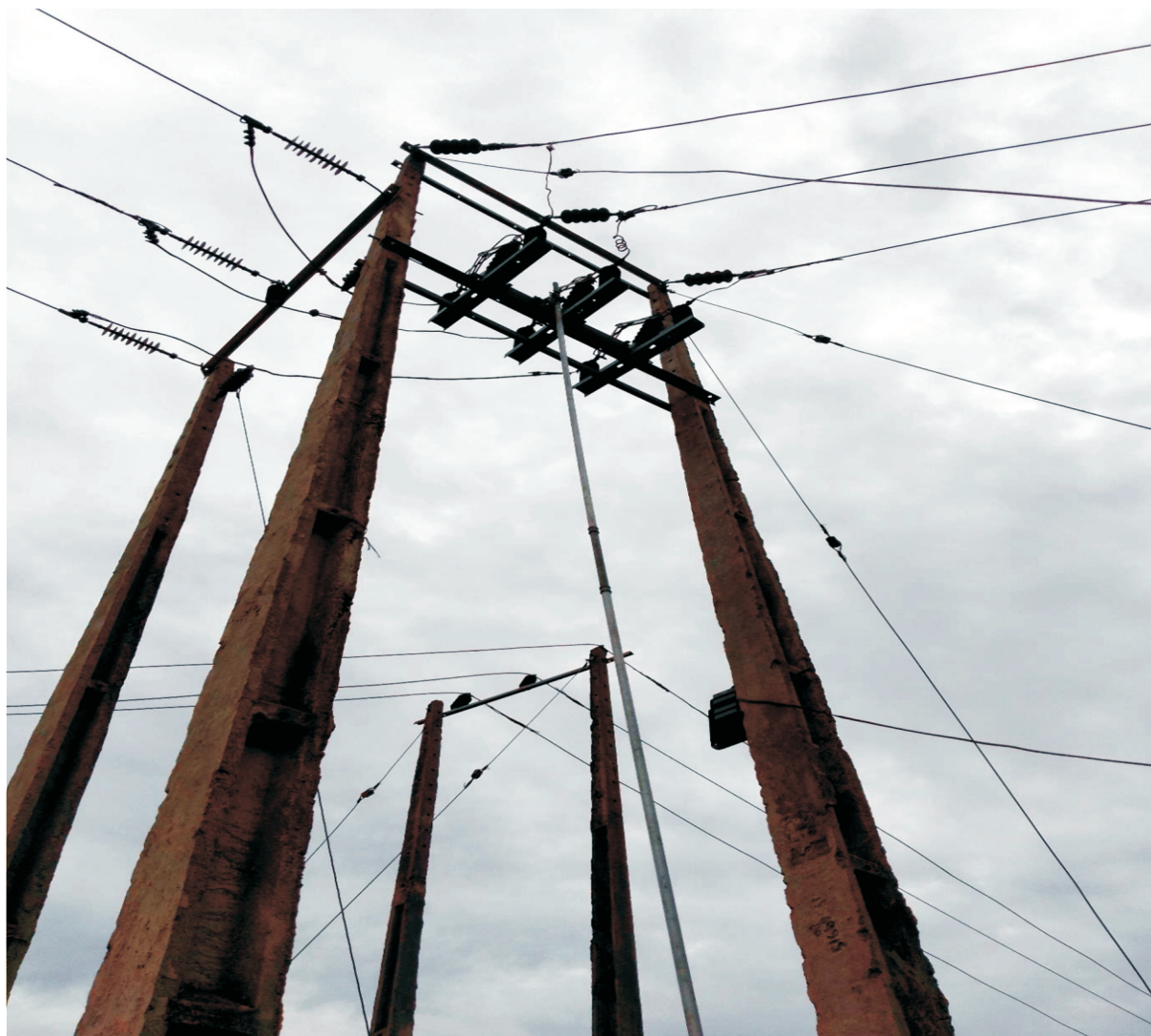
33kV Gang Isolator at University Main Gate
